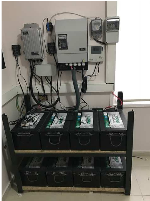
Figure 3.5. Off-grid inverter, sensors and batteries.
