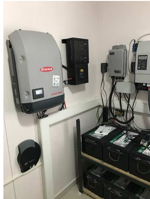
Figure 3.6. On-grid inverter with Solar-log.
